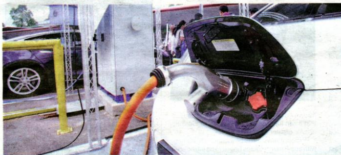
The first public solar Electric Vehicle (EV) Charging station in Malaysia at Ayer Keroh Overhead Bridge Restaurant (Southbound) on the North-South Expressway. PICTURES BY MUHAMMAD ZUHARI ZUBER
